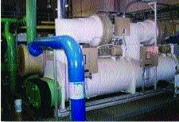
Trane centrifugal chillers in the chilled water plant at the University of Arizona, Tucson.
